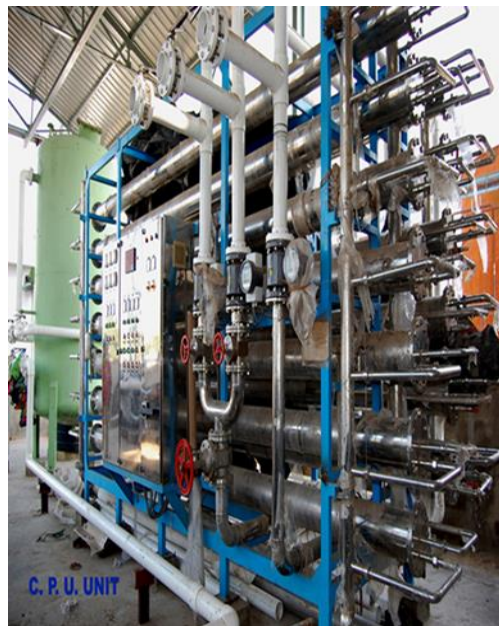
Condensate Polishing Unit (RO System)
