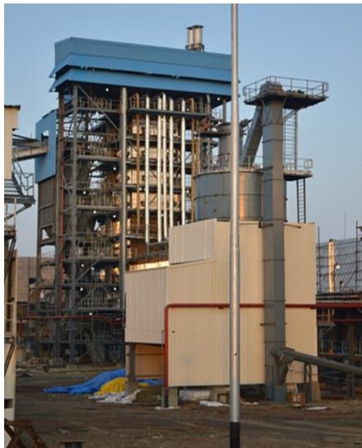
Incineration Boiler -40 TPH
