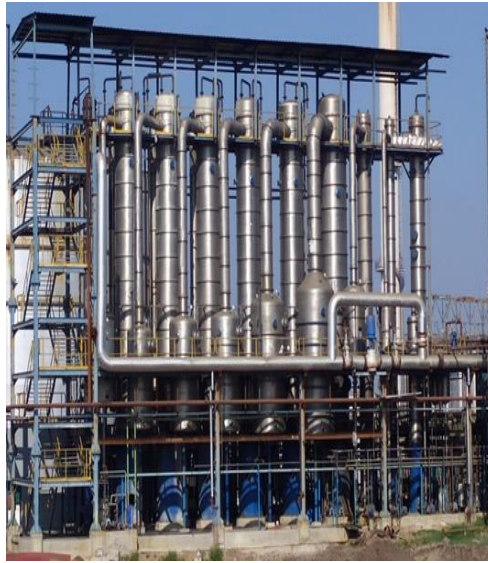
1 st Stage Evaporation (Falling Film
