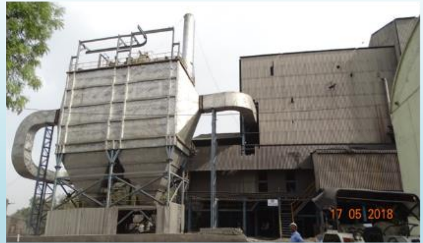
ESP provided for ISGEC Boiler (18TPH)
