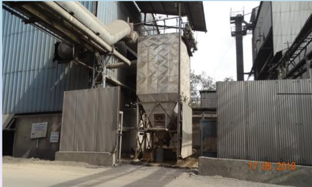
Bag filter for FBC Boiler (12TPH)
