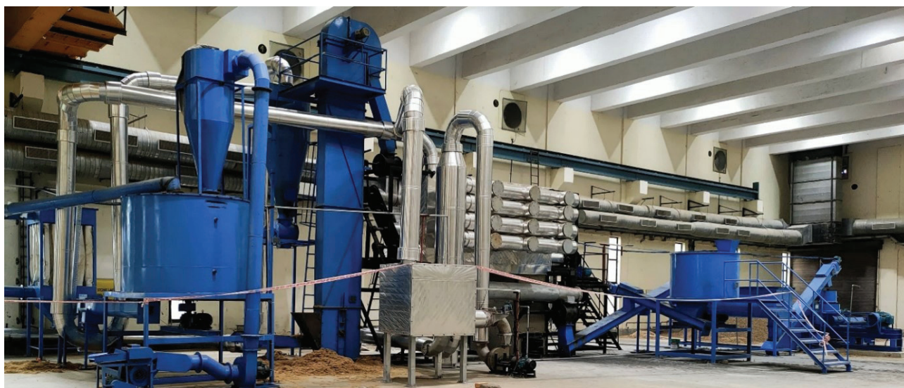
10 TPD Torrefied Pellets Manufacturing Plant at NTPC NETRA, Gr. Noida
