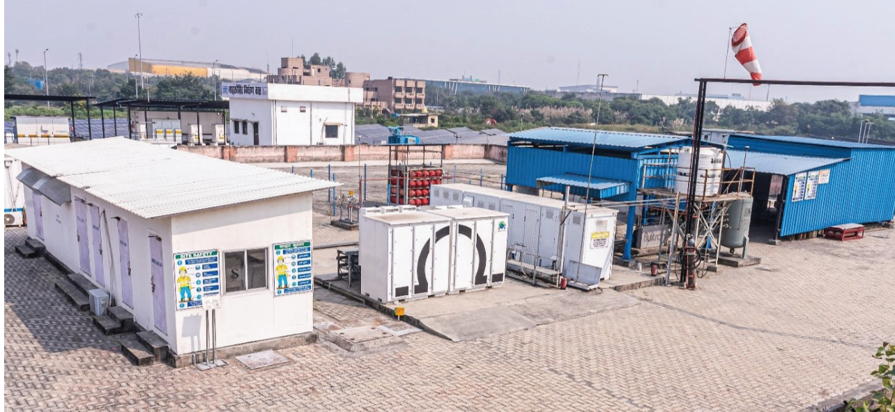
Sewage Water to Green Hydrogen Facility at NTC NETRA, Gr. Noida
