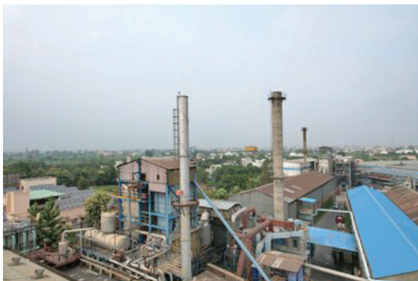
Biomass-fired boilers at MIL Hapur, operational since 2005 – burning rice husks and sawdust as direct fuel to generate process steam and thermal energy for manufacturing operations
