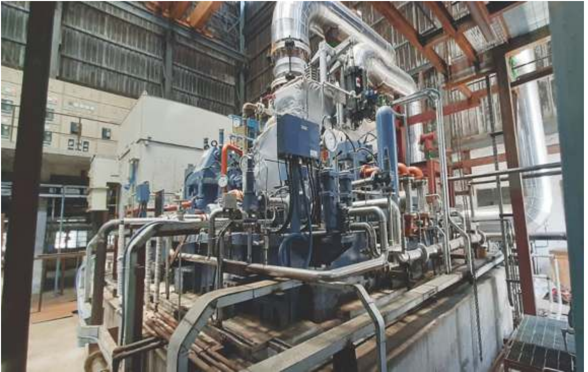
10 MW Turbine at Distillery Plant
