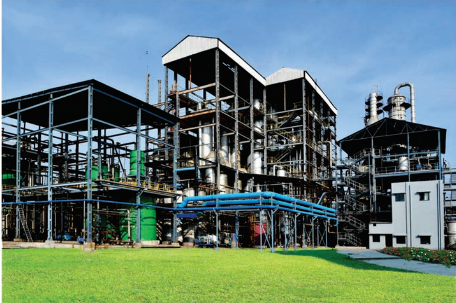
400 KLPD Distillery Plant
