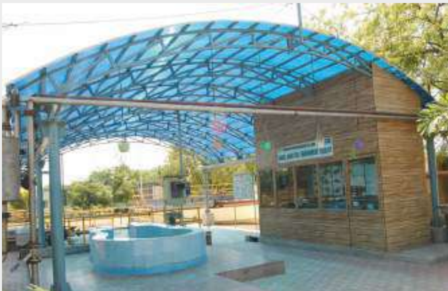
Effluent Treatment Plant
