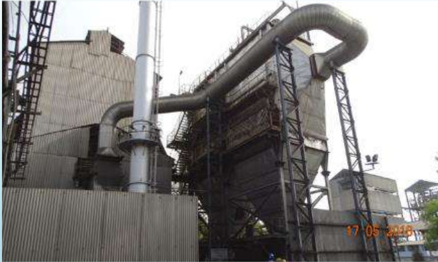
ESP for Thermax Boiler (18TPH)
