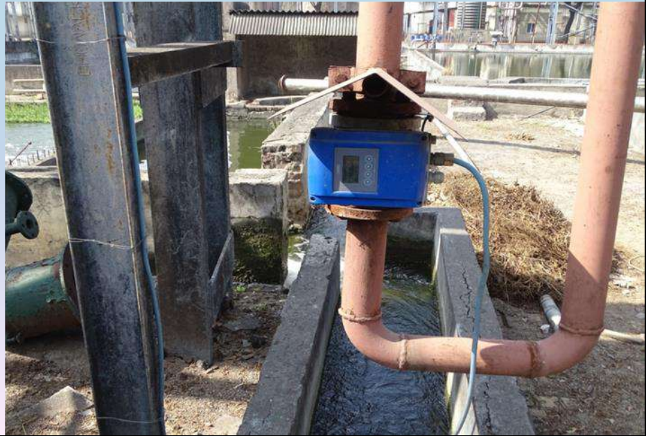
Domestic water supply
