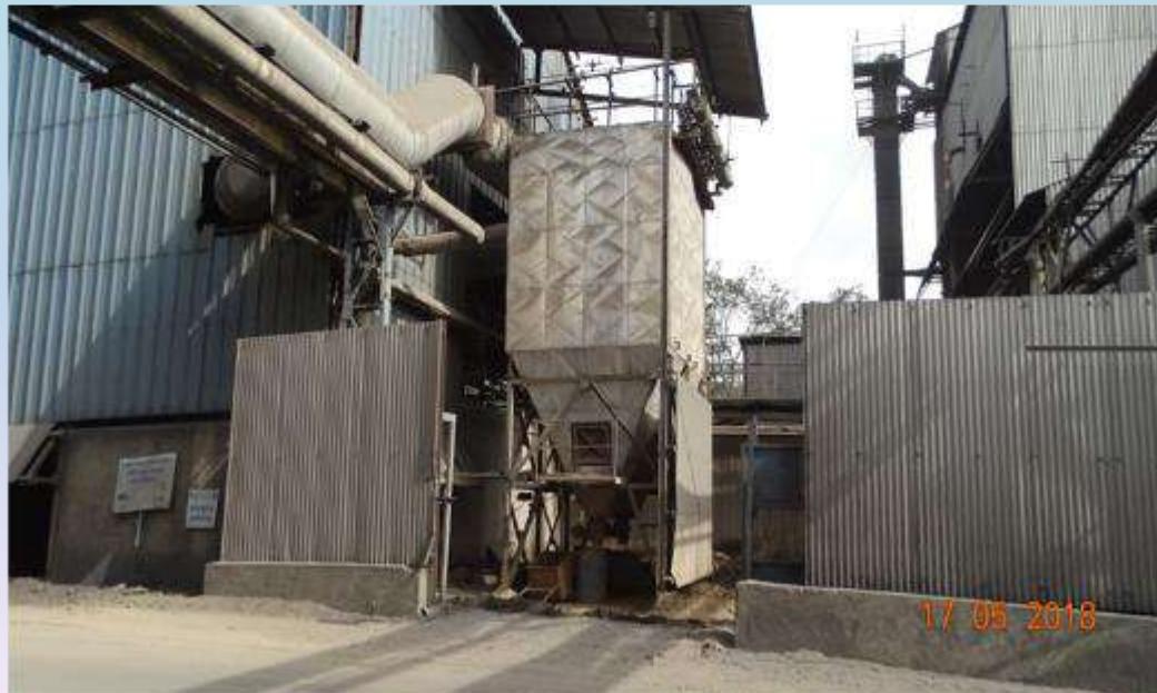
Bag filter for FBC Boiler (12TPH)
