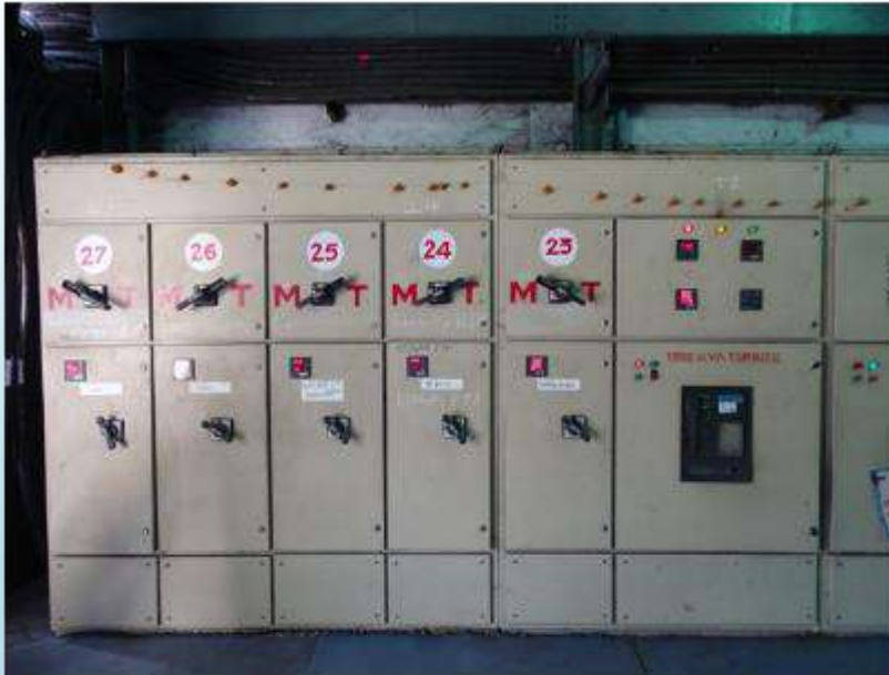
Pollution Control Facility
