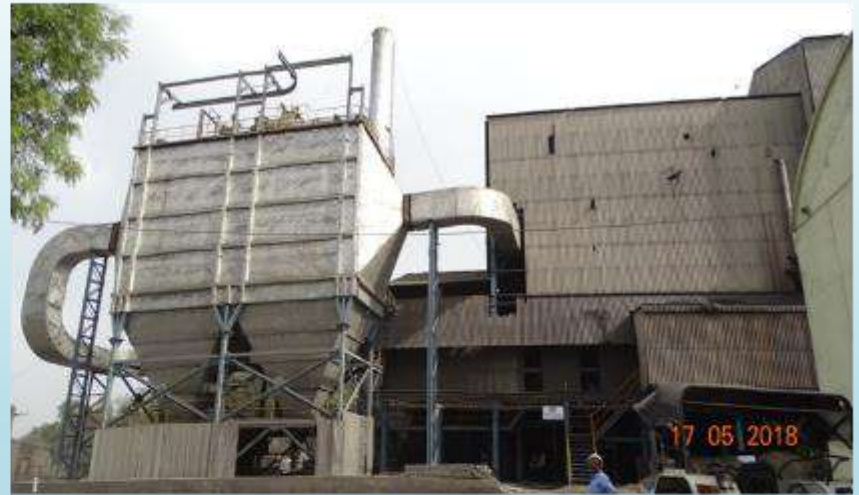
ESP provided for ISGEC Boiler (18TPH)
